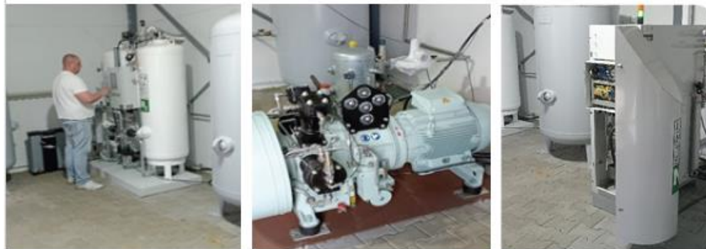
Nitrogen-generating plant equipment
